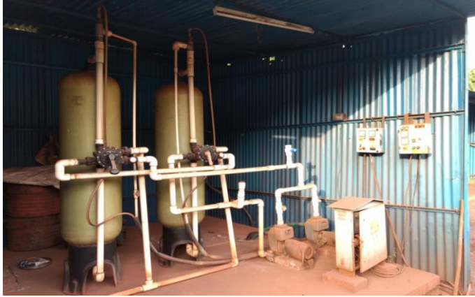
Photo-11: STP for treatment of Domestic Waste Water (Ultra Filtration Unit)
